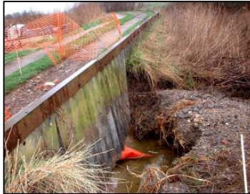
Washout under crest piling
