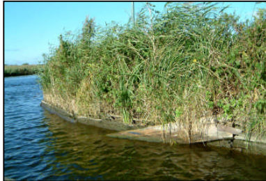
Lost or damaged topboards Examples of areas requiring maintenance.
