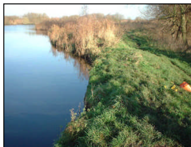
Erosion pocket before construction
