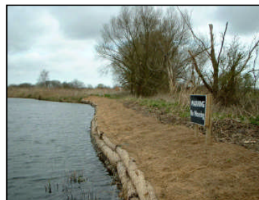
Gabions topped with reed rolls and backfilled with clay, covered with a Coir blanket.
