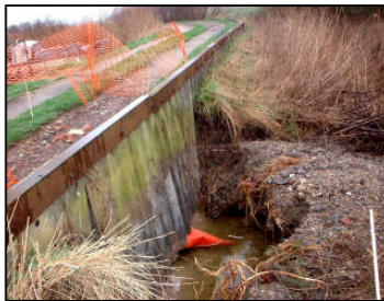
Washout under crest piling
