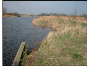
Scour pockets and narrowing road
