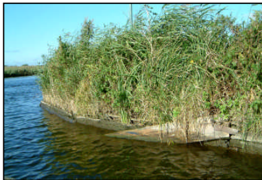
Lost or damaged topboards Examples of areas requiring maintenance.
