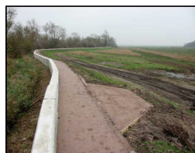
Footpath enhancement at Rockland (joint venture with Broads Authority and Norfolk County Council)
