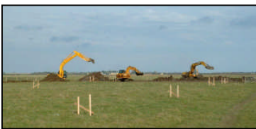
Early stages of set back bank with line and slope profiles visible in foreground
