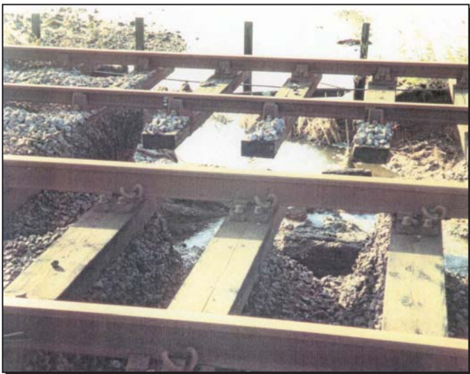
Breach under railway line - 1993
