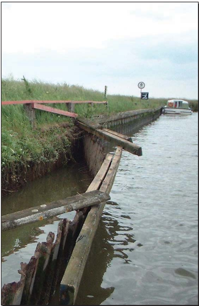
Failed piling on the River Waveney
