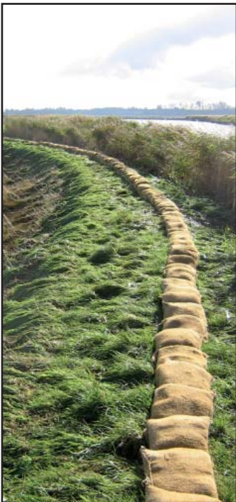
Length that overtopped, November 2006
